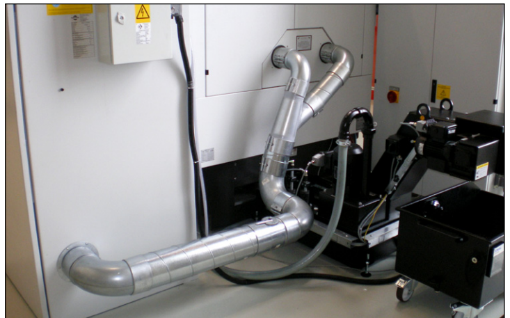
Connection ductwork to machine tool
