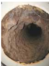
Prior to cleaning
