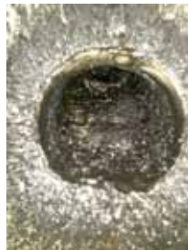
Prior to cleaning
