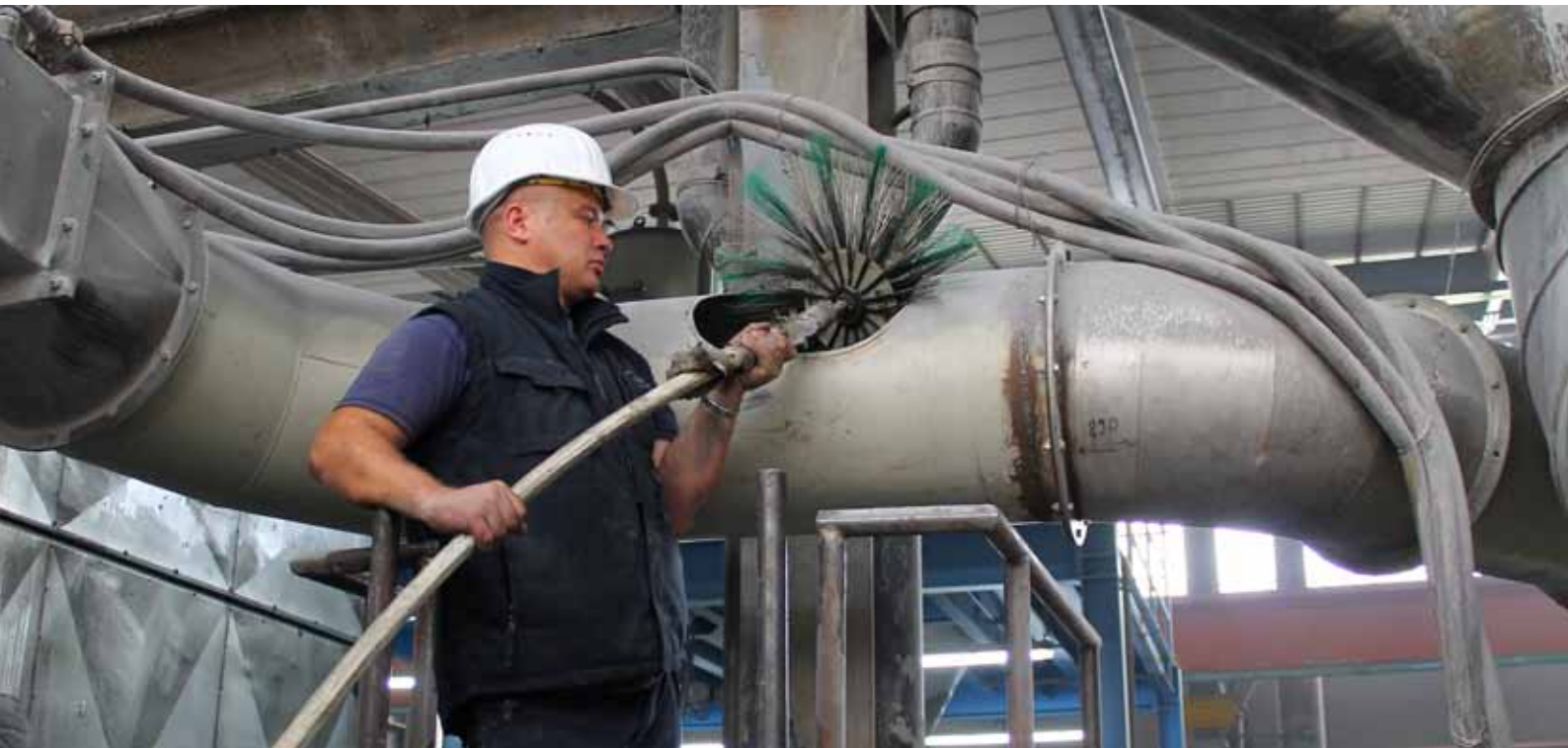
Clean ductwork contributes to continuous separation efficiency and frequently reduces the risk of fire.
