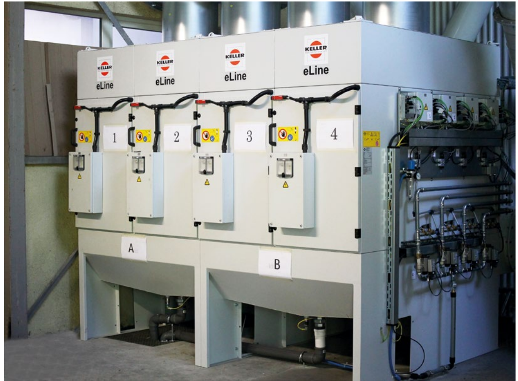
The four eLine modules clean the air so well that it can be recirculated into the plant. "This will have a noticeably positive effect on heating costs next winter," says Dr. Michael Haas.
