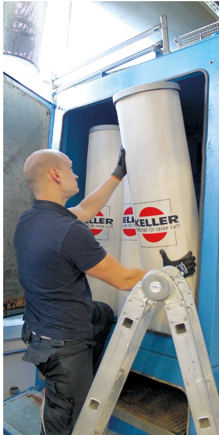
At regular intervals, a service technician from Keller Lufttechnik inspects the two oil mist separators which collect the flue gases, filter out foreign substances from the air, and exhaust them from the plant.
