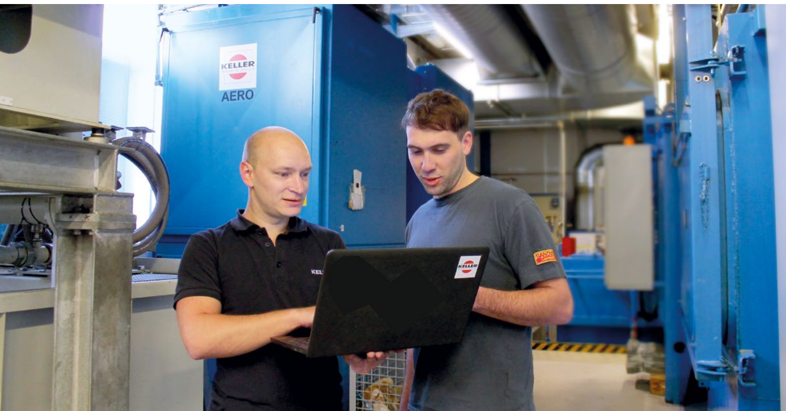
Stefan Heimerdinger (right) takes the maintenance of the system-critical separators at his hardening shop very seriously. With the peace-of-mind service agreement with Keller Lufttechnik, he benefits from regular maintenance and professional cleaning of his extraction systems.
